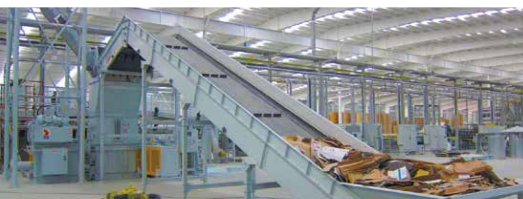
7 Scrap Handling Conveyors
